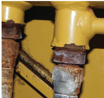
Figure 4: Corrosion migration to adjacent components
